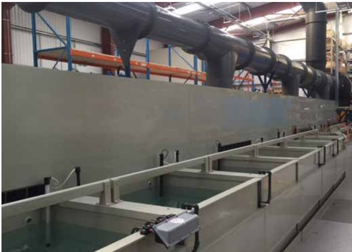
Electro polishing plant
